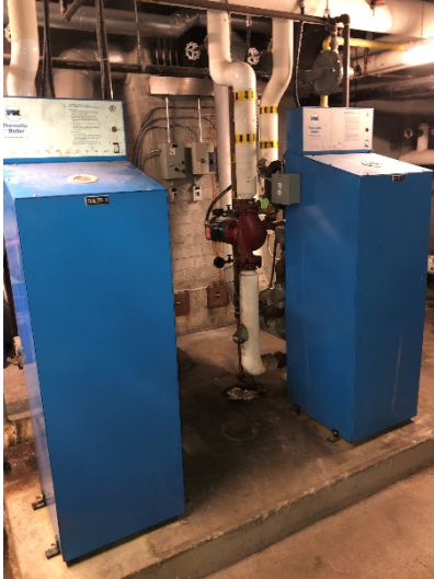
Before (Mid Efficient Boilers at Leigh Elementary)
