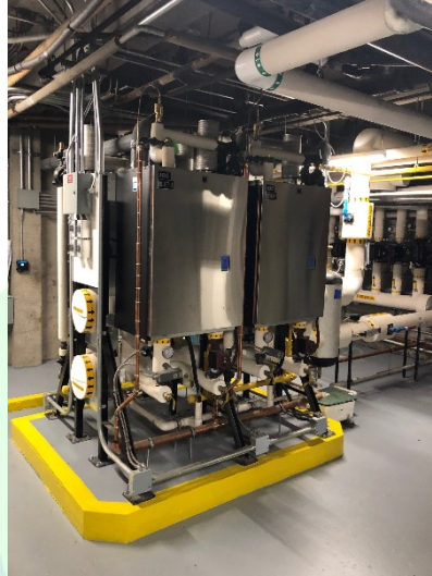
After (highly Efficient Condensing Boilers at Leigh Elementary)
