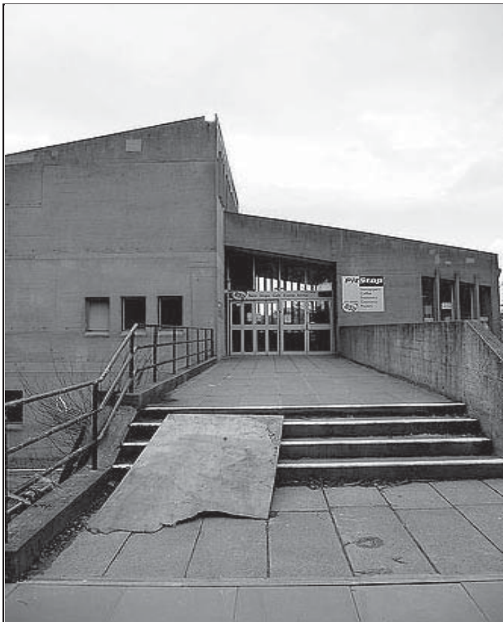
Above left: Does that look like wheelchair accessibility to you?
